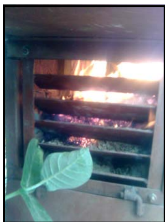
Combustion chamber for loose biomass
