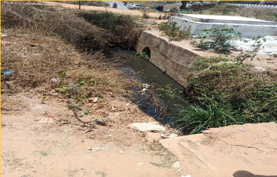
Figure 5.2 Greywater outlet, Vapasandra
