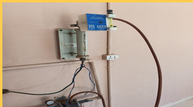
Figure 3.7 Chlorine dosing tube
