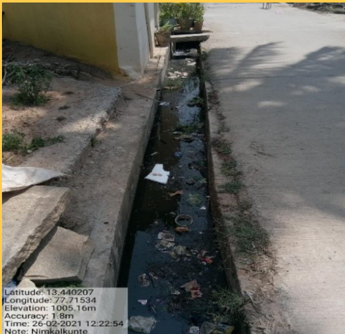
Figure 4.4 Dumping of solid waste in open drains.
